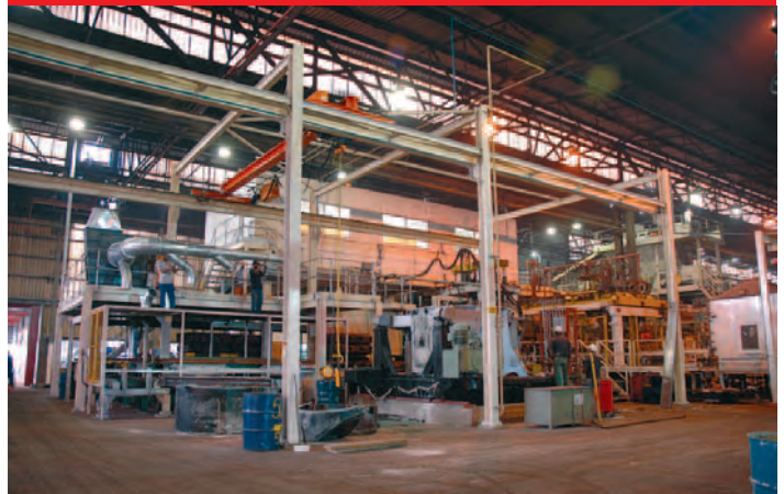
Moulding Line, installed
