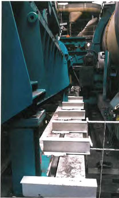
Illustration of the required detailed engineering in order to perform installation in an operational foundry within designated area
