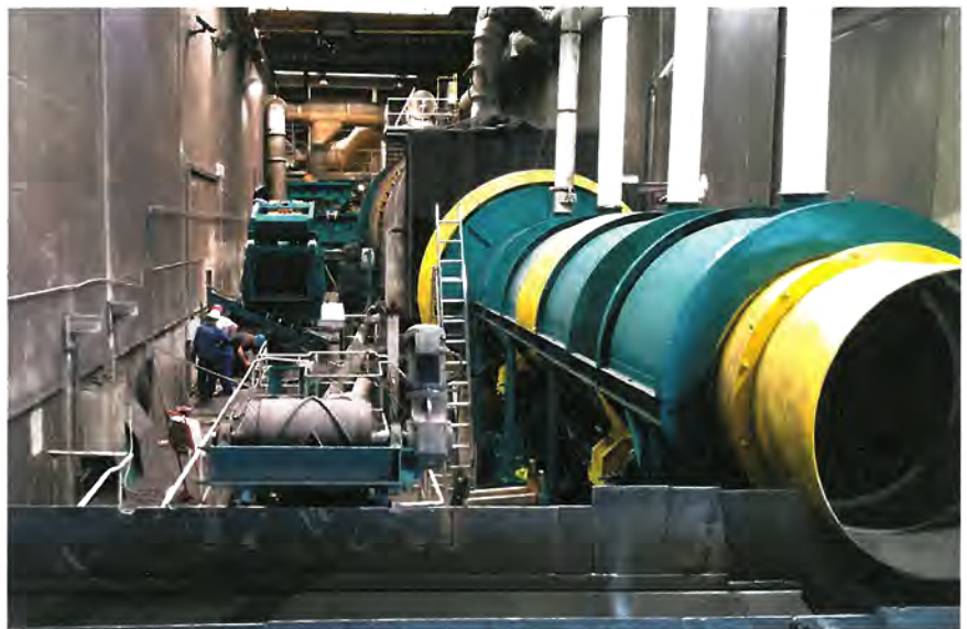
Installation works in a small area in which a gentle shakeout, conveyors and the new screening system are to be positioned next to the installation of a new drum (Photos: Gemco)
