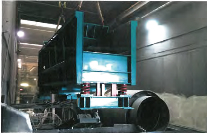
Positioning of the gentle shake out equipment
